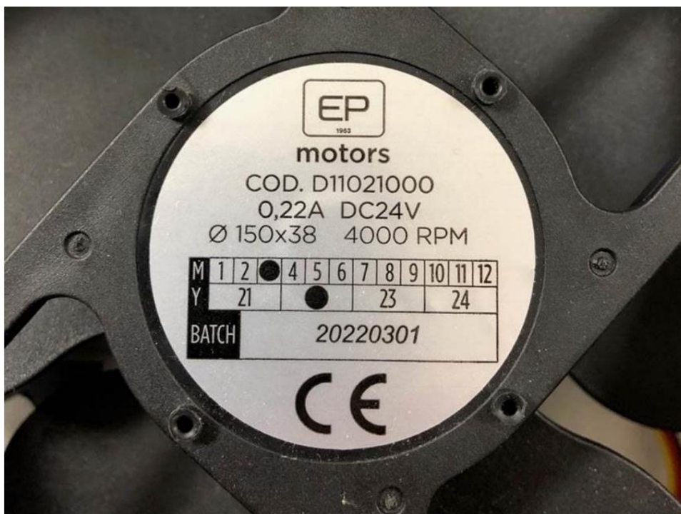
Figure A-9: Fan nameplate
